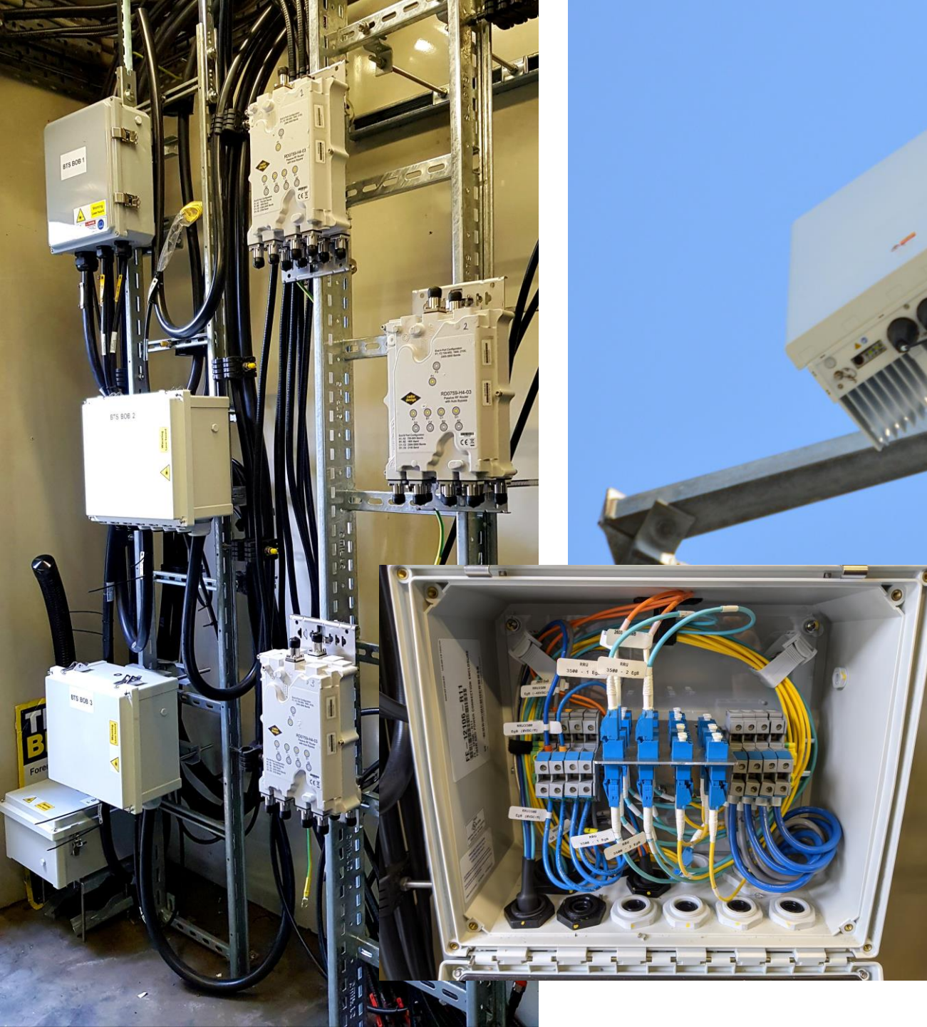
Fibre to the tower (FTTT) - fronthaul
